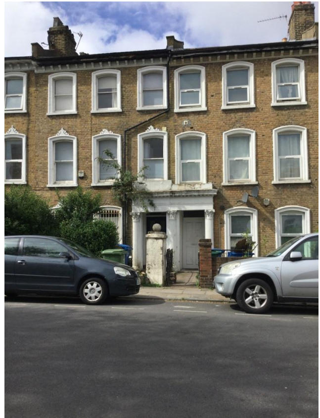
Figure 18 Unsympathetic alterations (loss of historic boundary treatment, satellite dishes, security grilles and uPVC windows)
